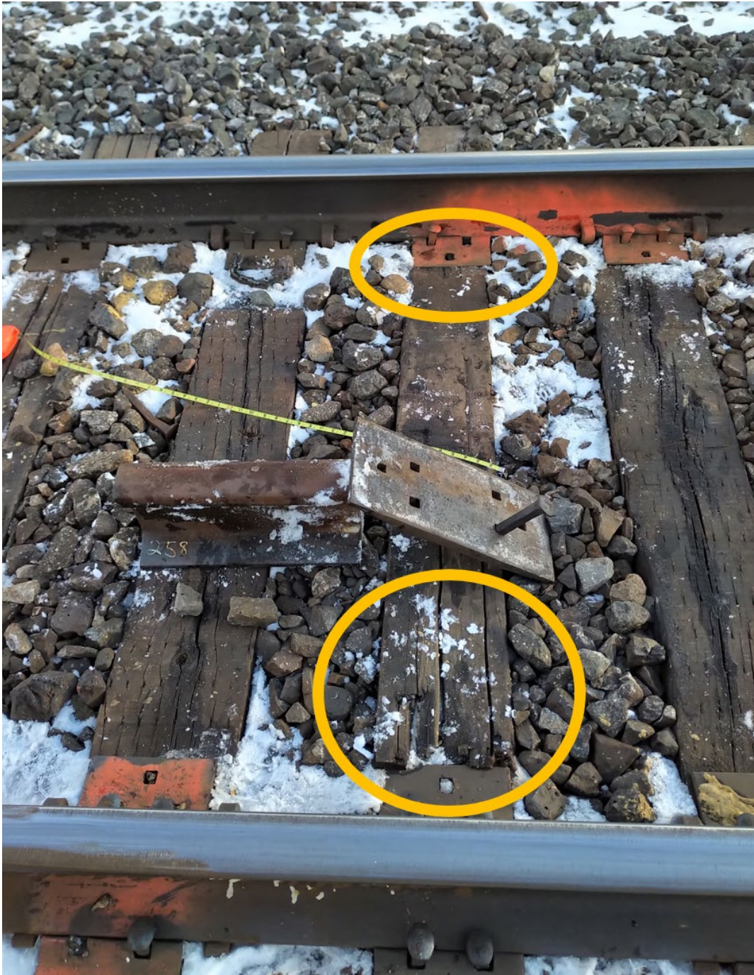
Figure 5. Tie at the west end of the replacement rail showing cracking along the length of the tie and wood decay under the tie plate (Source: TSB)
