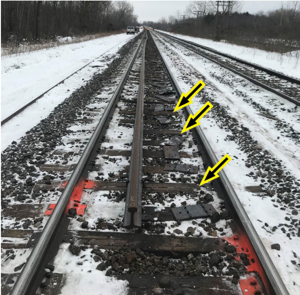
Figure 3. West end of replacement rail, facing east, showing some ties without tie plates on them (Source: CN, with TSB annotations)
