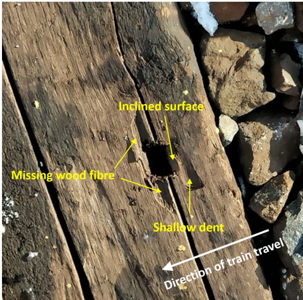
Figure 4. Tie at the west end of the replacement rail showing the spike hole and the crack in the tie (Source: TSB)
