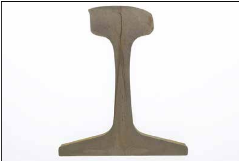
Figure 18. Rail cross-section taken 3 inches west of the thermite weld, with physical separation in the head and web streaking
