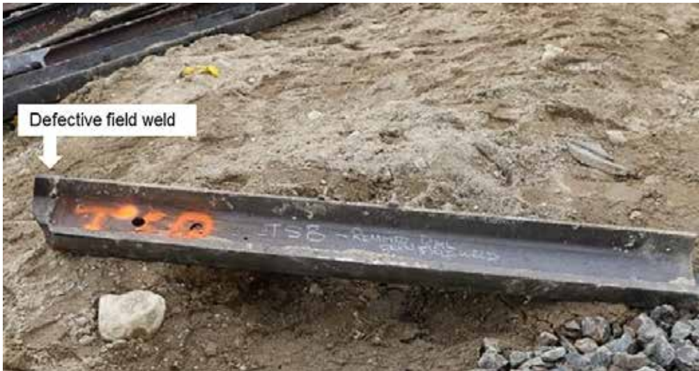
Figure 5. The 68-inch-long section of rail with defective field weld
