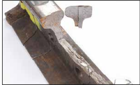
Figure A1. Vertical split head defect observed in head and web of rail
