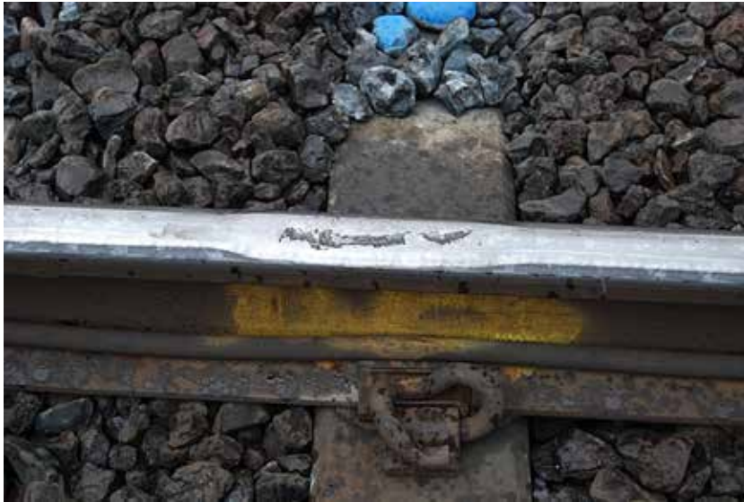
Figure 12. Photograph of a typical localized surface collapse
