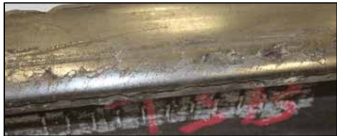
Photo 7. Head checking on the gauge face of the rail
