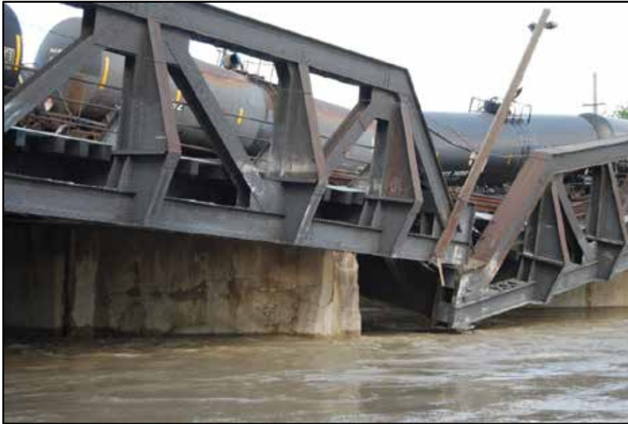
Photo 1. The bridge failure and derailment (with river flow left to right)
