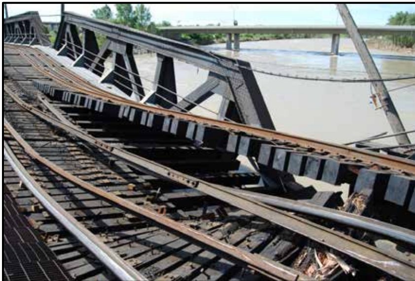
Photo 4. Bridge deck at Pier no. 2, showing tracks P1 and P2 after removal of the tank cars, with Ogden Road Bridge in the background
