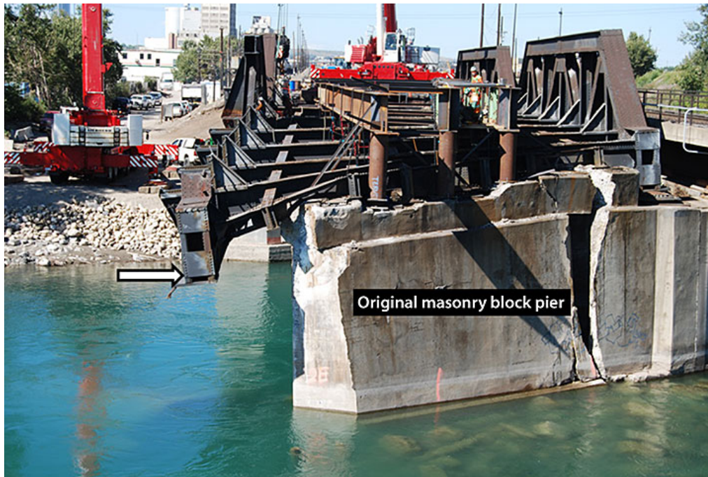
Photo 7. An arrow indicates the unsupported span bearing. (River flow is right to left.)
