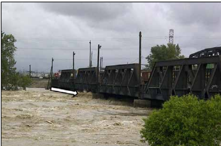
Photo 6. Bonnybrook Bridge (from downstream) on 21 June
