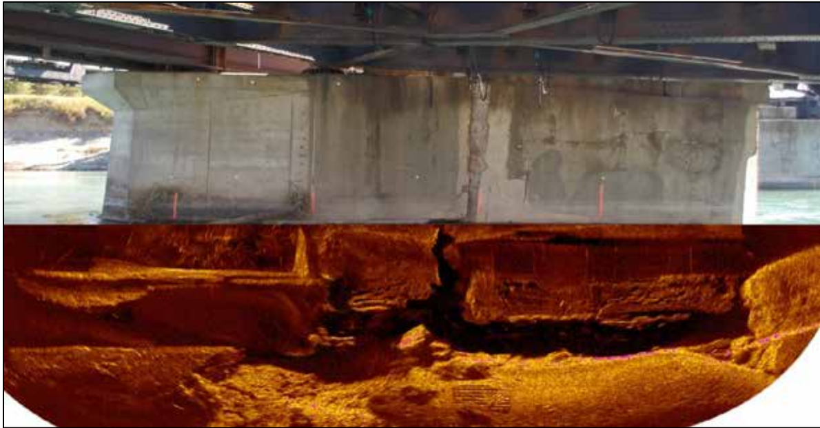
Photo 10. Sonar image of the west side of Pier no. 2, showing the extent of scour
