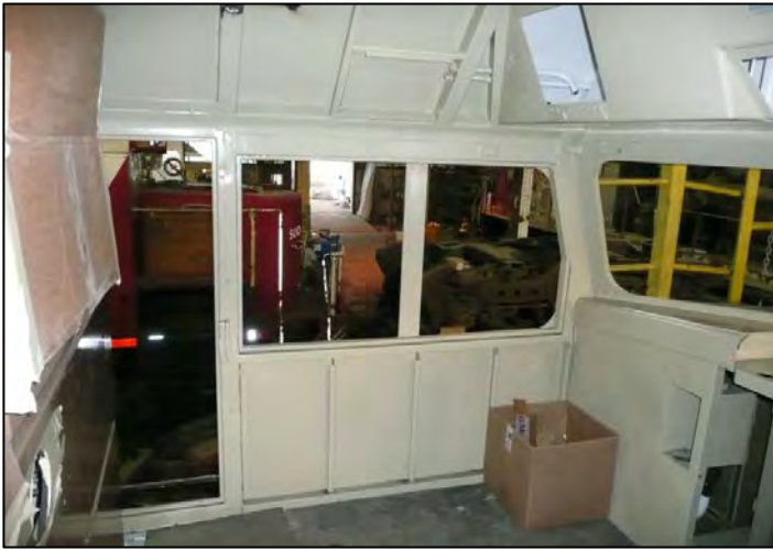
Photo 9. Exposed cab interior structure, conductor side (source: TSB)
