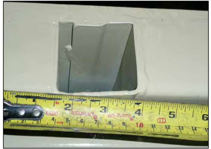
Photo 10. Tubing used for roof framing structure. Roof sheeting at top of photo (source: TSB).
