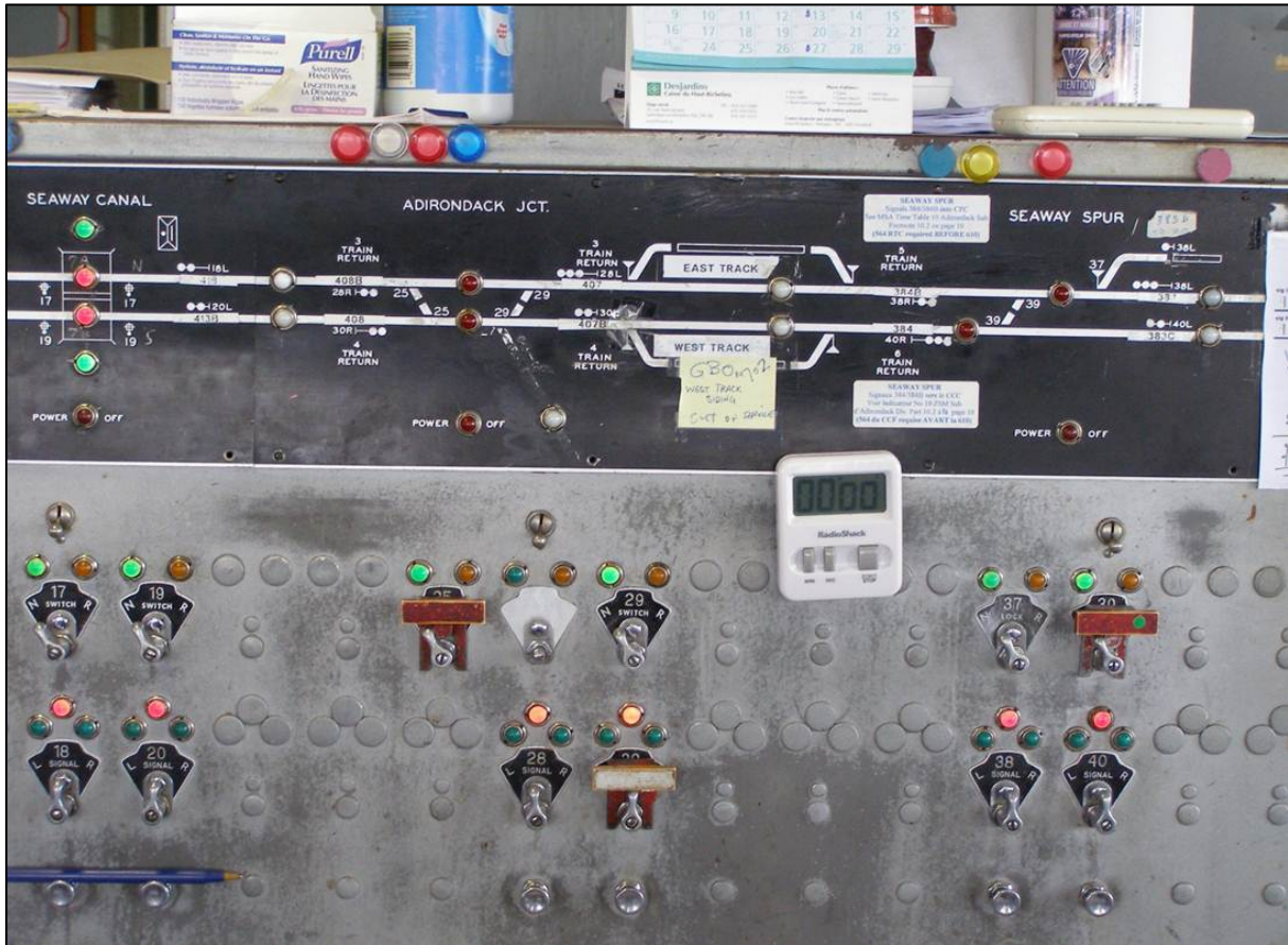
Photo 1. Traffic control board for Seaway Interlocking
