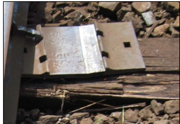
Photo 3b. View of tie plate showing rotation and polish from rail cant and base rotation
