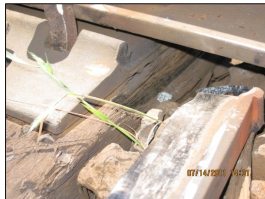
Photo 3d. View of tie and plate showing low rail field side plate cut, rail seat polishing and tie splitting
