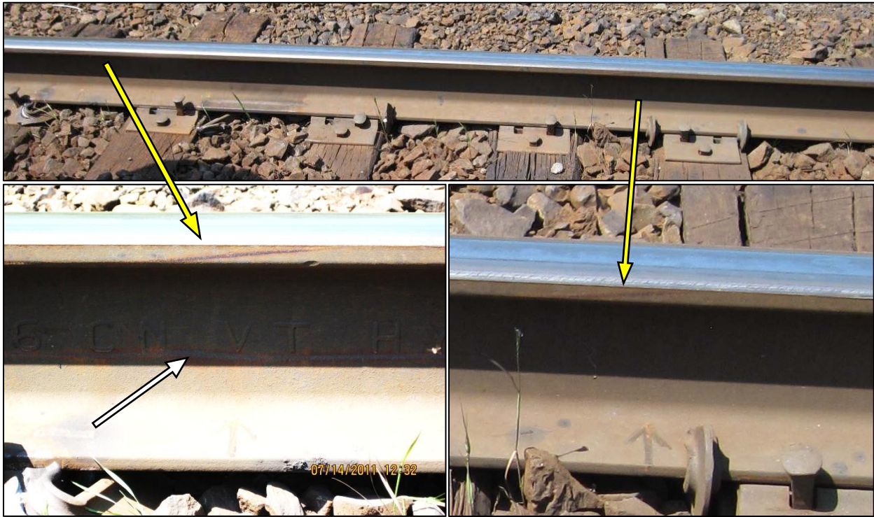
Photo 2. Photo of low rail gauge side at POD. Yellow arrows point to rim marks where the L4 wheels (left close-up photo) and L3 (right close-up photo) dropped into gauge. Note the wheel rim mark (white arrow) in the rail web just inside the margin of the rail head shadow.
