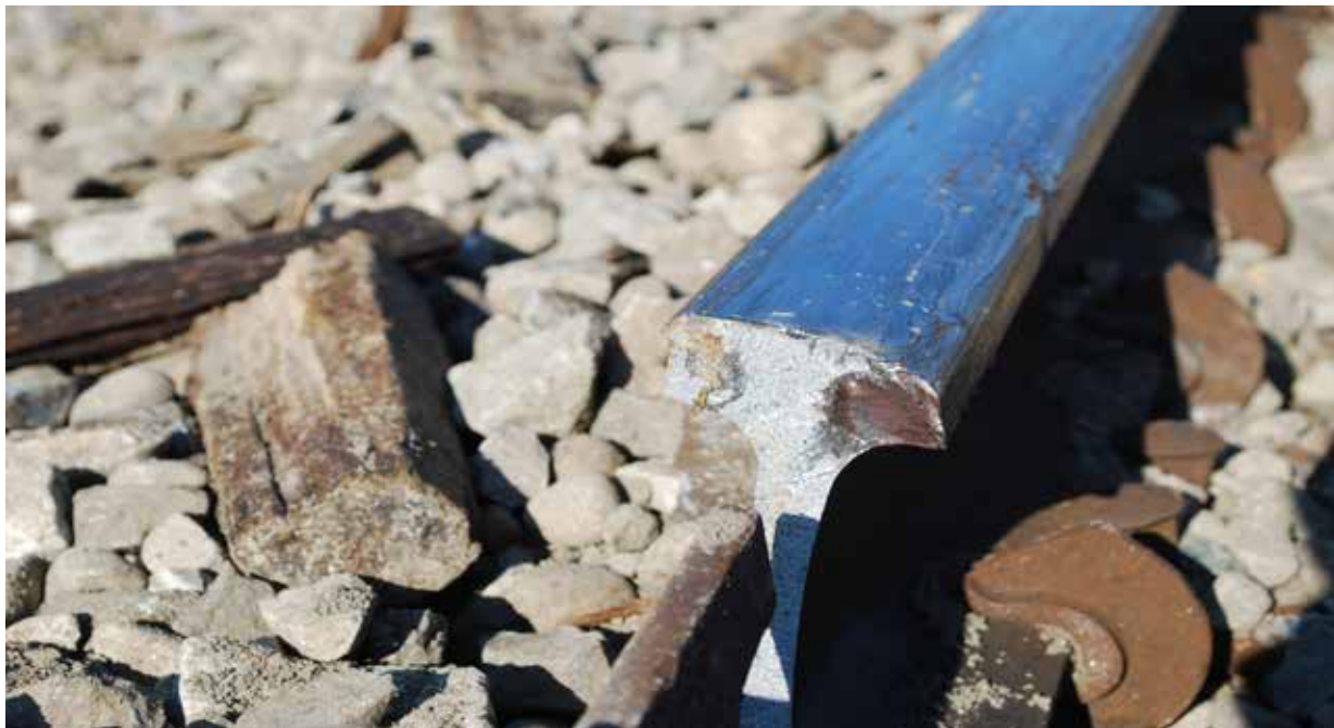
Photo 2. Broken rail with 2 transverse defects
