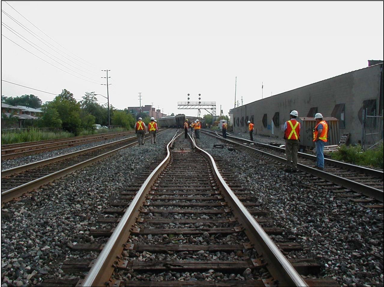
Photo 2. Track buckle at turnout (Mile 6.0)
