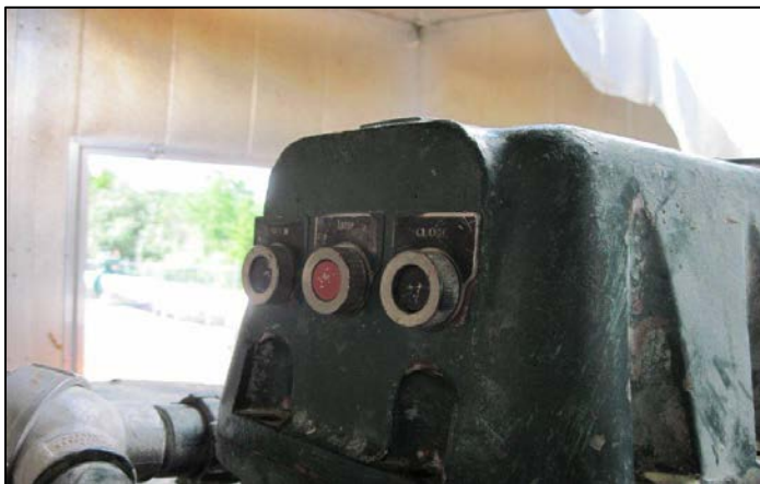
Photo 4. Manual control switches
