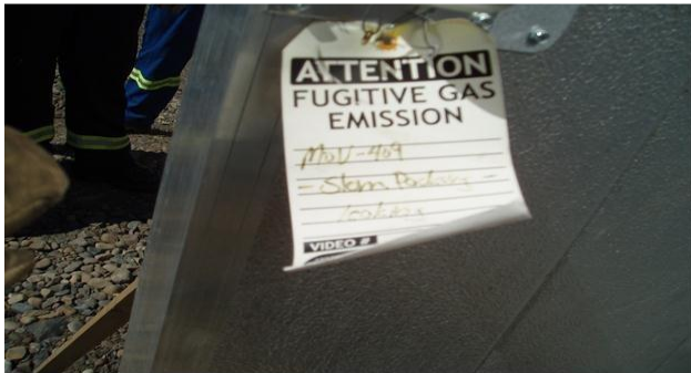
Photo 1. Fugitive gas emission (FGE) tag for MOV-0409
