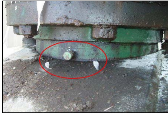
Figure 5. Bull plug installed on MOV-0409
