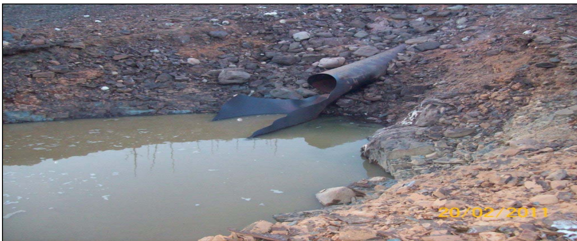
Photo 3. Upstream line-break section of Line 100-2
