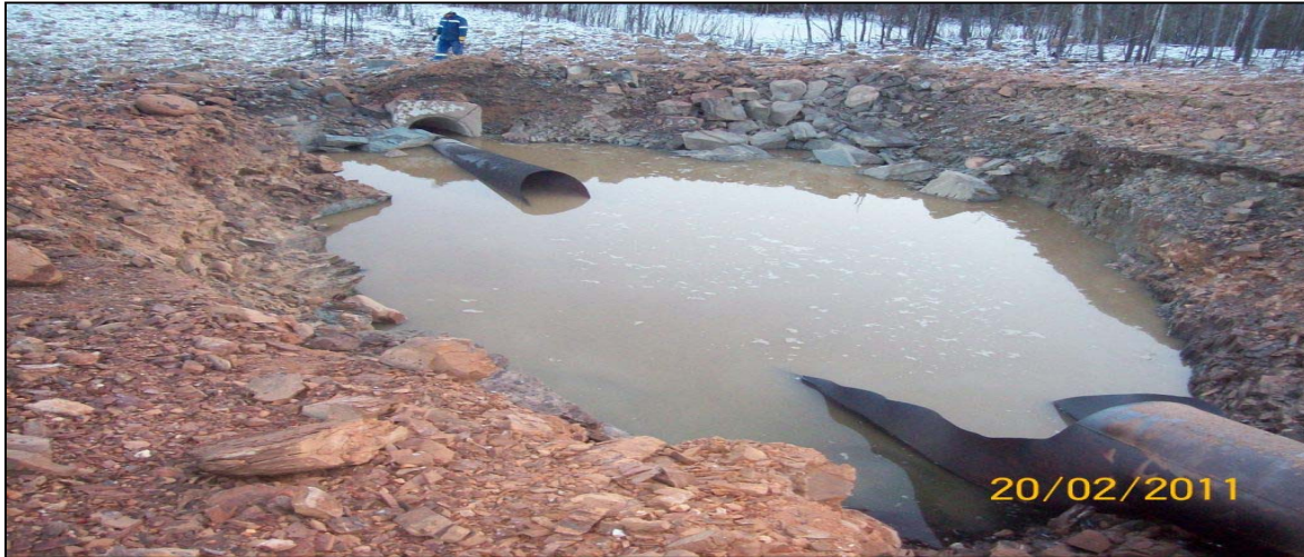
Photo 2. Downstream line-break section of Line 100-2 (top of photo)
