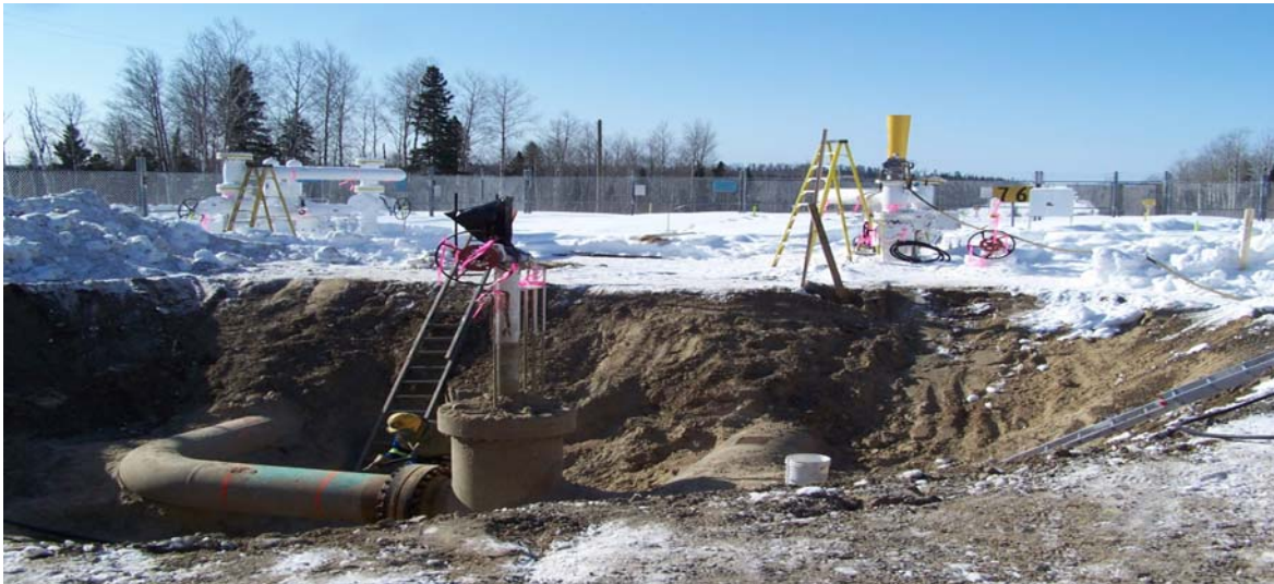
Photo 4. Cross-over valve and associated piping between lines 100-2 and 100-3
