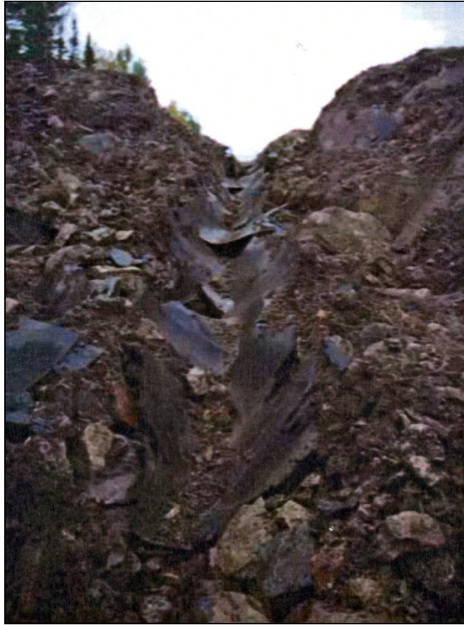
Photo 5. Line 100-1, disbonded exterior coating found in the ditch after the rupture.
