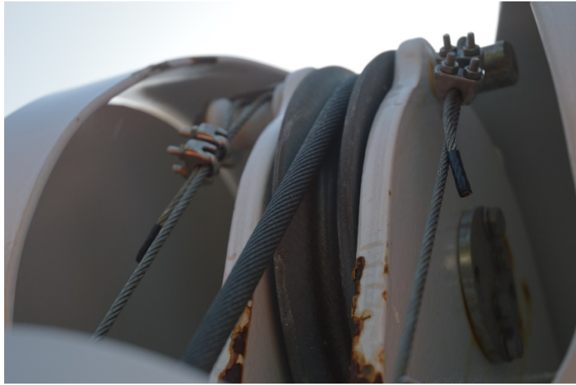
Figure 5. Correct rigging of limit switch, as shown on the Queen of Capilano, a similar vessel in the BC Ferries fleet (Source: TSB)
