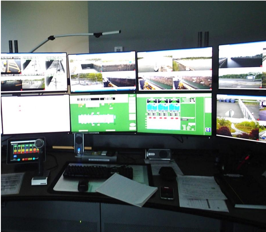
Figure 3. Lock operator workstation
