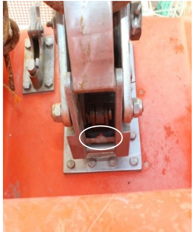
Figure 10. Lifeboat forward release hook in the closed position, with on- or off-load release mechanism lock-position indicators aligned (white circle). Operator's view would be obscured by deck design. (Source: TSB)
