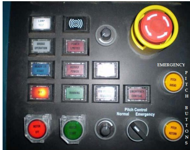
Photo 2. Pitch control panel
