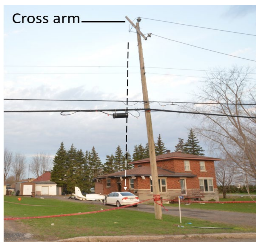
Figure 1. Hydro pole and dotted line showing the angle of the pole in relation to the automobile (Source: TSB)
