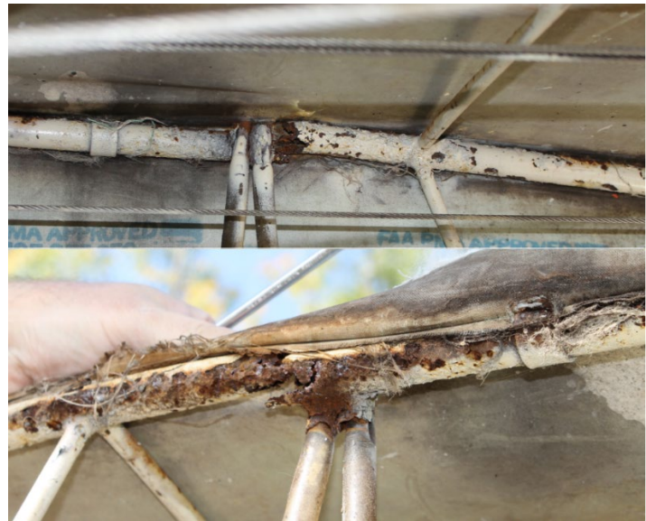
Figure 3. Photos of the steel tube structure below the battery that were severed by corrosion, taken from 2 different angles (Source: TSB)
