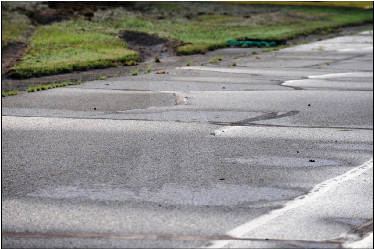
Photo 4. White steam-cleaned marks
