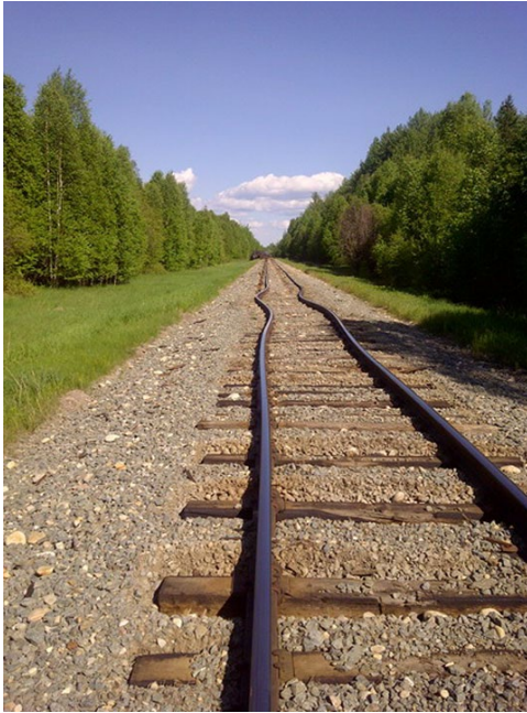
Figure 6. Track buckle (Source: TSB Railway Investigation Report R14E0081)
