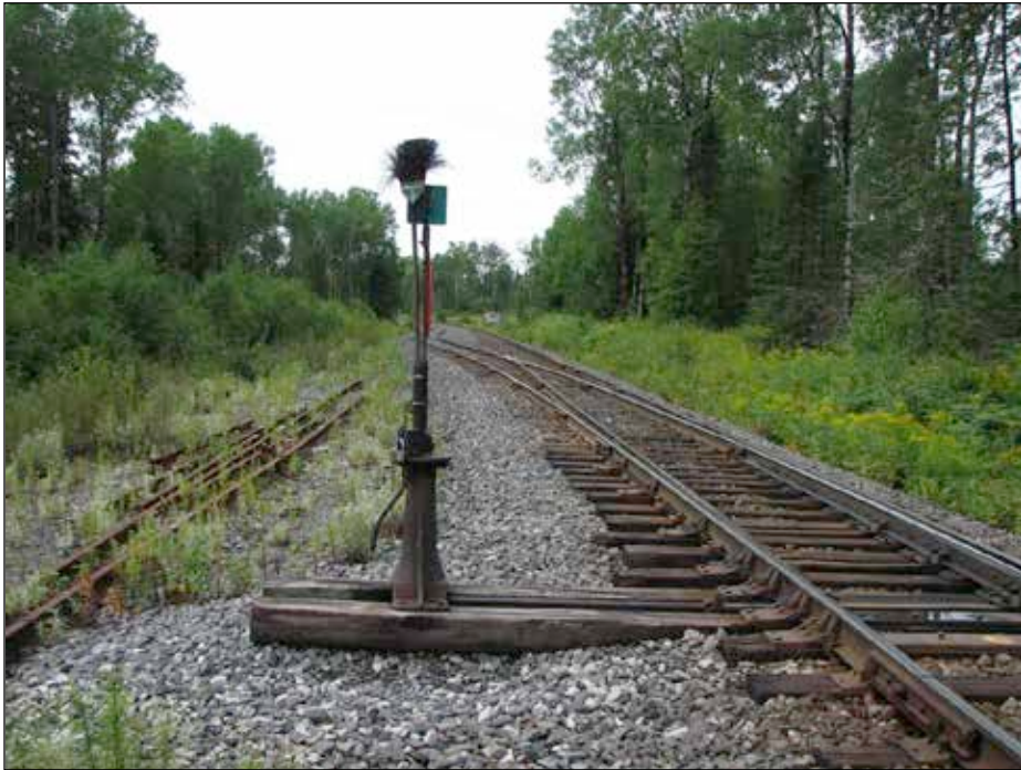
Photo 1. JM33 turnout switch stand in normal position
